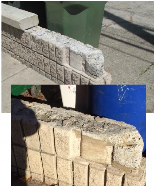
Before: Broken blocks, missing cap
